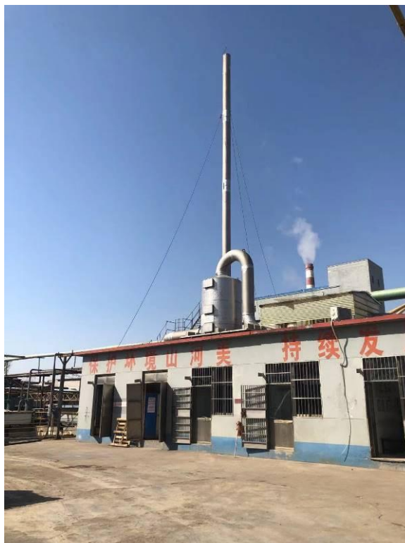
污水站臭气排气筒 ( h=30m/r=0.6m )
